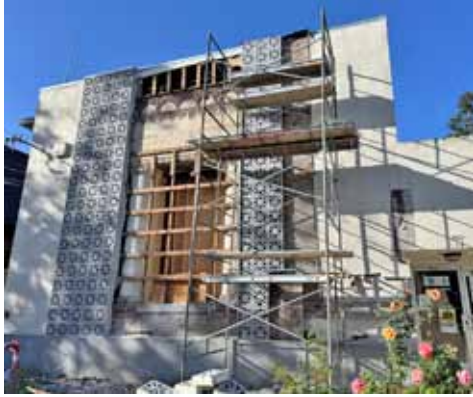
Removal of the false front begins exposing the original entrance and details on the facade.
