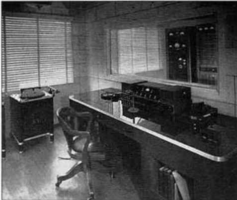
control room c. 1930s
